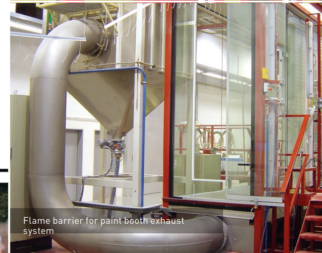
Detection of fire in paint booth
